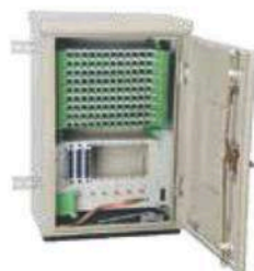
96 Core Fiber Optic Cabinet (PLC Tray type)
